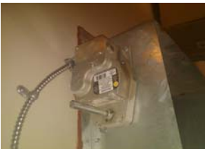
Honeywell. Like for like replacement.
