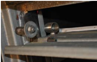
Above. Negator spring is attached to the blade and a post coming from the damper frame. The one above is broken.
